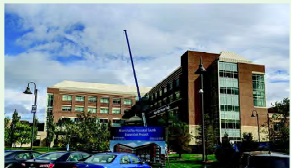
MVHS $60 million renovation and expansion construction project by ESI Electrical Contractors, Inc..
